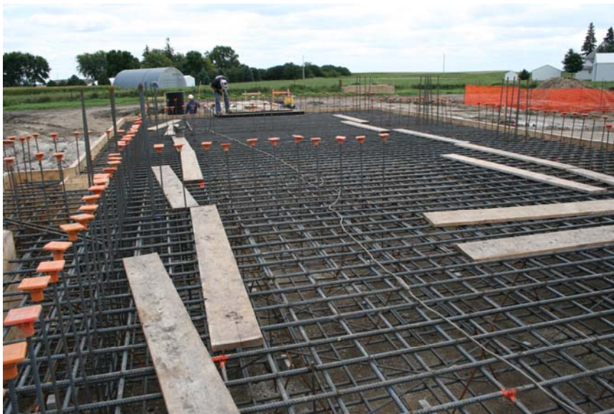
An up-close view of the re-bar being used in the floor pad of the mill.
