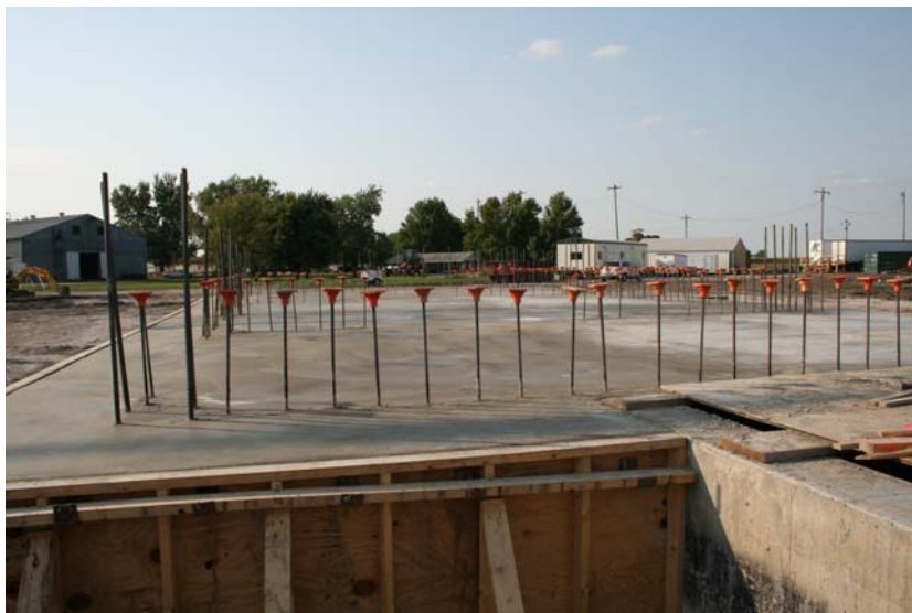
The finished concrete mat pad of the mill. Ready for the slip forms next.
