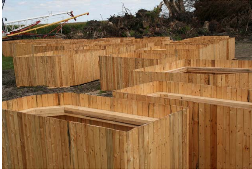
Multiple wooden slip forms ready to go to the pad for each bin of the mill.
