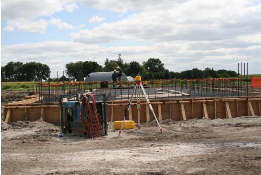
A view of re-bar being set up for the floor pad of the mill.
