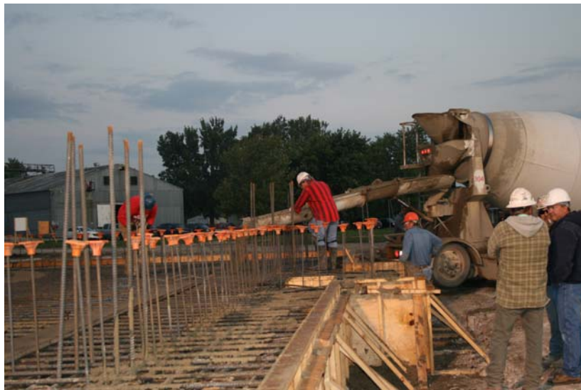
The first load of concrete for the mat pad. Picture taken at 6 am.
